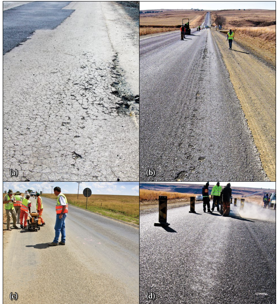
Figure 2 Examples of premature failures at case study sites: (a) general surface failure, (b) rutting and aggregate loss in wheel tracks, (c) bleeding in wheel tracks, (d) bleeding in isolated areas
